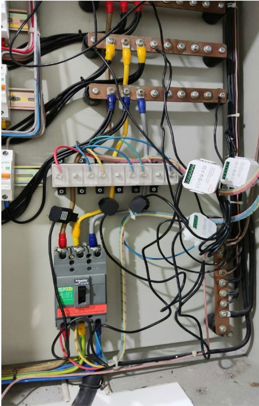
Fig. 3 The clamp power energy monitors installed in the 4th floor control box
